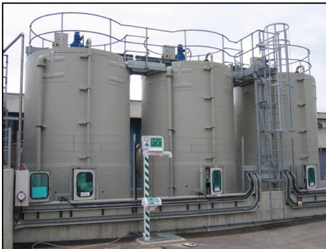
3 x 30m 3 storage tanks for water treatment manufactured using Crystic 397PA
